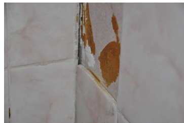
Asbestos contained sheeting and adhesive behind tiles
