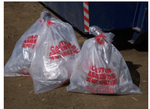
Example of asbestos double wrapped.
