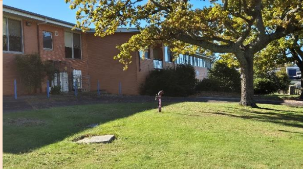
Existing fire plug
