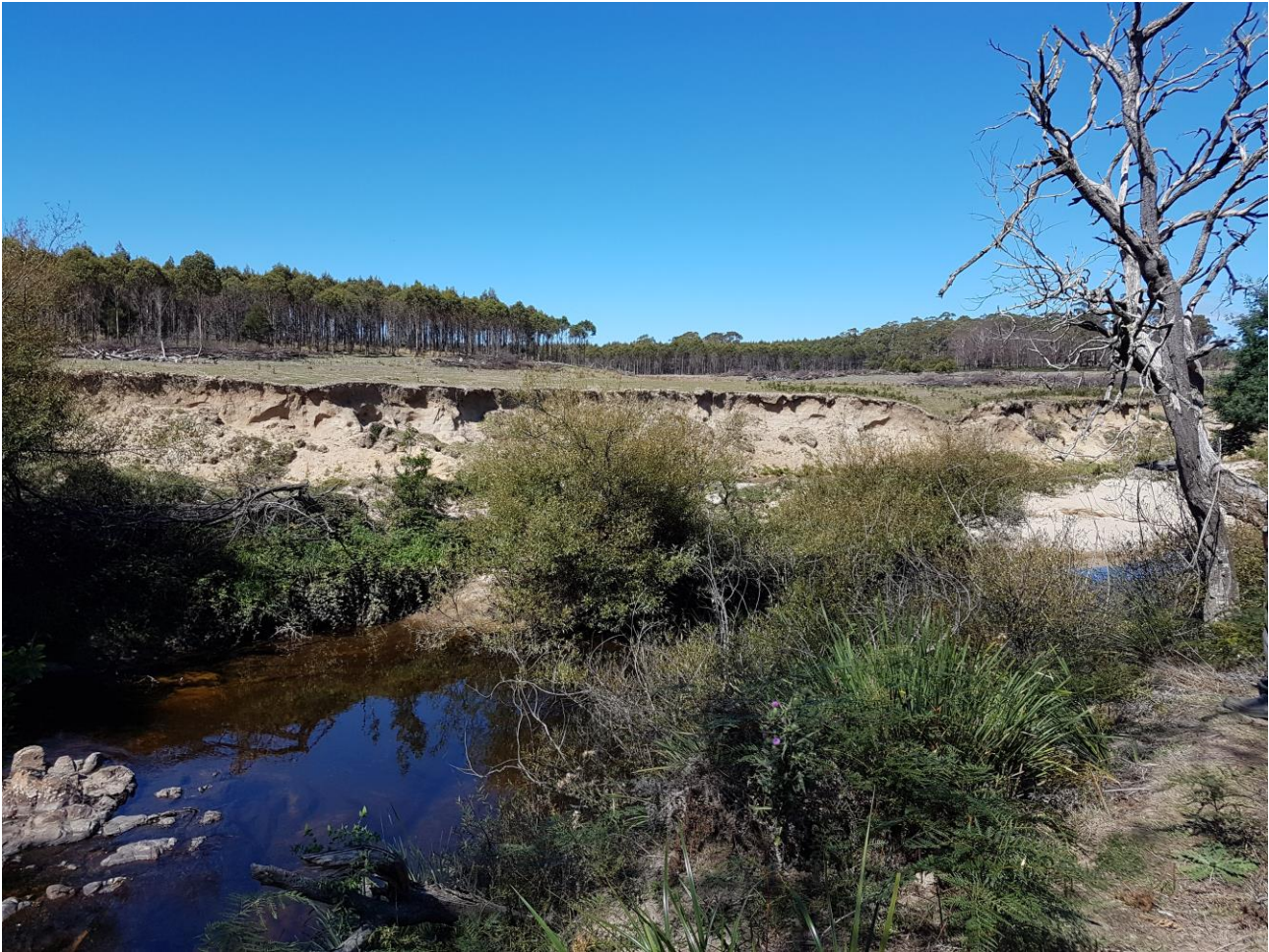
FIGURE 2-11 EXTENSIVE BANK EROSION APPROXIMATELY 8M HIGH, OVER A 400M LENGTH.
